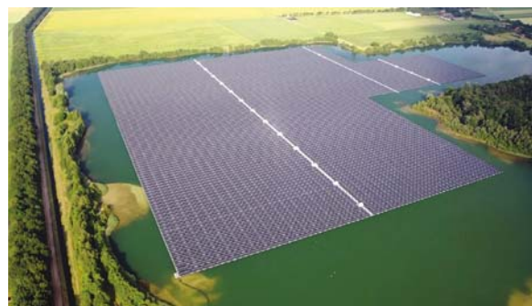
The 41.1MWp Sellinger plant was constructed on a former sand extraction lake.
