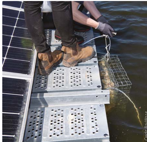
“Bio huts” are being submerged beneath the floating solar panels at the floating PV park Bomhofsplass, filled with seashells to potentially encourage marine life and greater biodiversity
