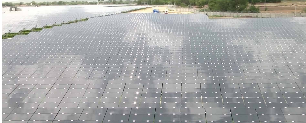
This project in Telangana, India, features First Solar modules. Thin-film technologies had a strong share of the Indian market share in the early part of the last decade, but they have since lost ground to rapidly expanding Chinese crystalline silicon manufacturers.
