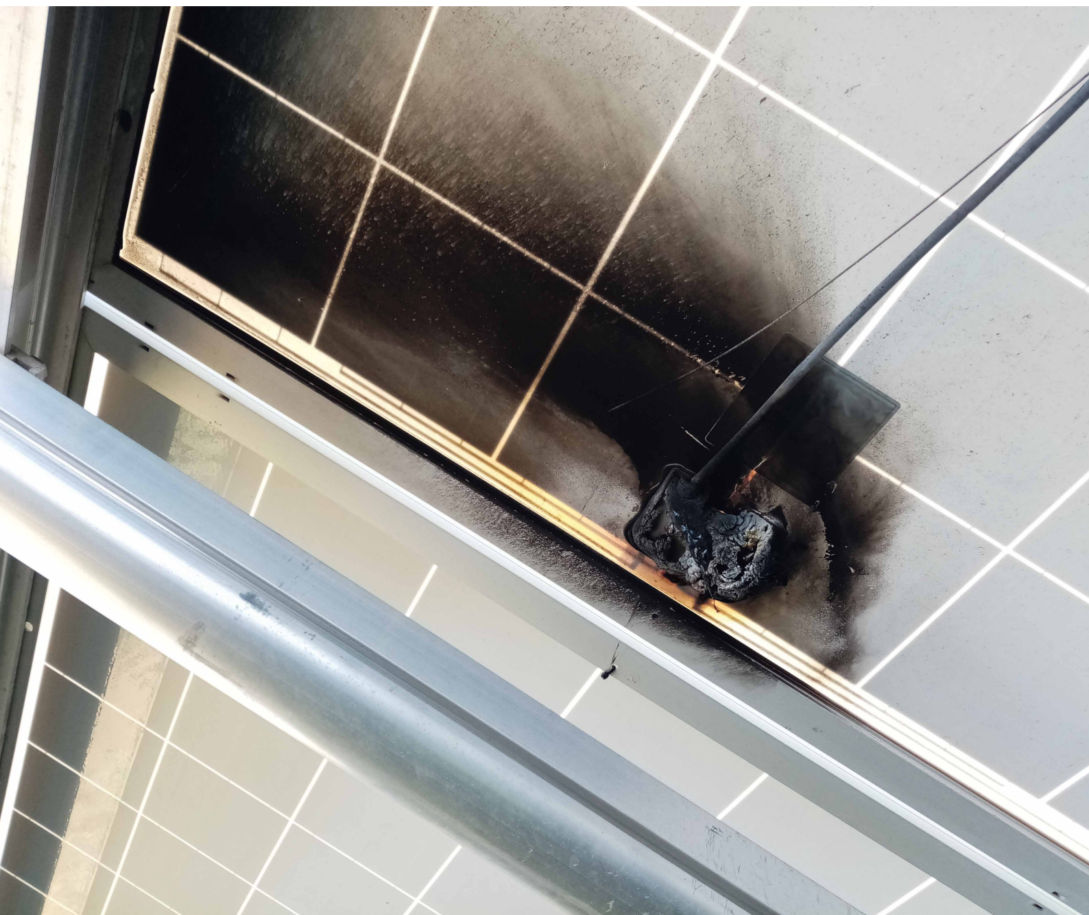
Junction box defects can lead to heat buildup, with damaging consequences for the module.
