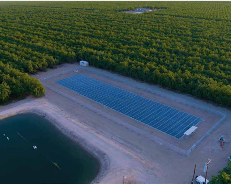
Installation demonstrating Erthos' approach in Bakersfield, California.
