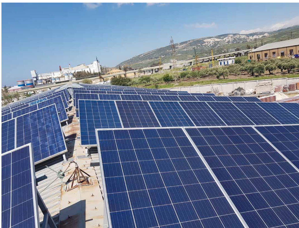
This 220 kWp rooftop PV system in Beirut’s port was destroyed by the blast on Aug. 4, 2020, just 10 days after being commissioned.
